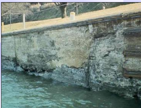
Crumbling lock wall, Lower Mon 3, opened in 1907
