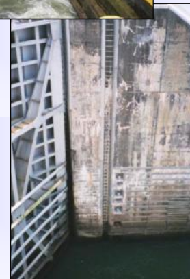
Concrete deterioration at Chickamauga could result in lock failure
