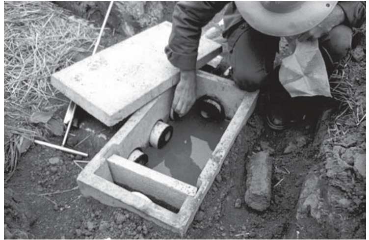
Figure 4-8. Distribution box with adjustable weir outlets
