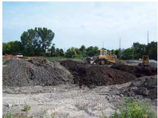
Debris piles on south side of site
