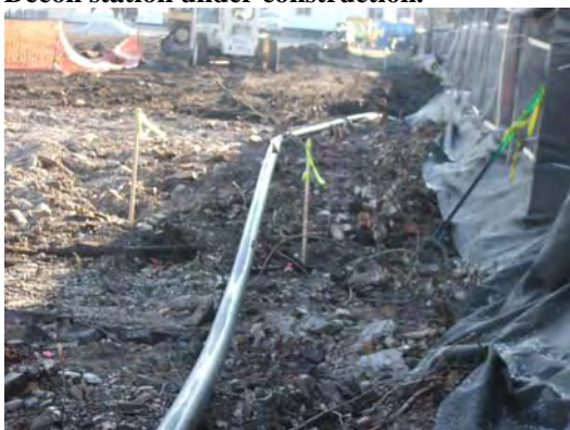
Envirocon's slurry piping.
