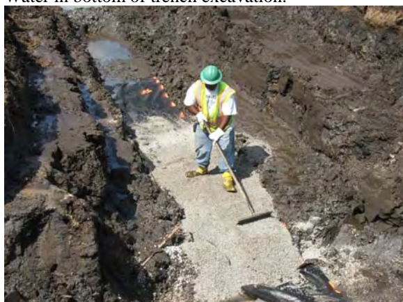
RW Collins placing CA-6 stone in trench and grading As per spec.
