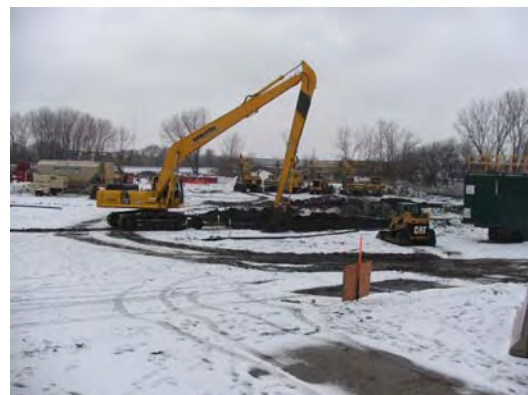
Final position of slurry wall excavator at end of day. Approx. 10+00 Station non structural.
