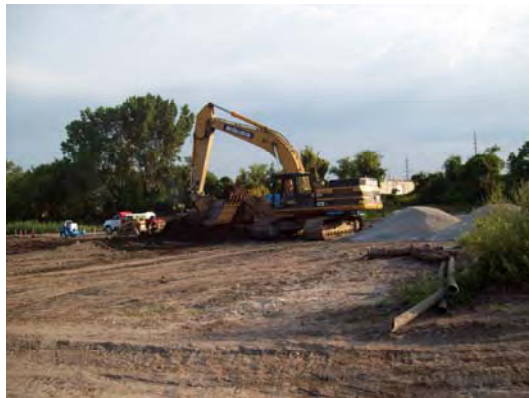
RW Collins moving debris and bulk material from the river edge to the south side of property
