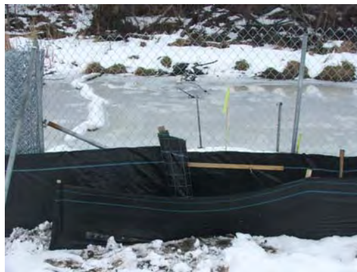
Northwestern silt fence.
