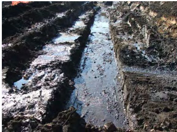
Water in bottom of trench excavation.
