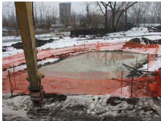
Secure slurry pond.
