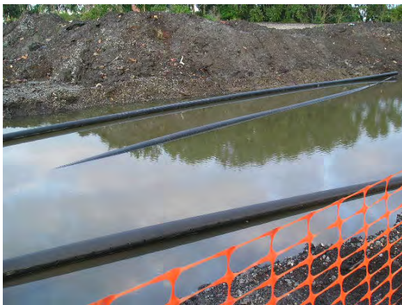
6" HDPE piping along collection trench #1.
