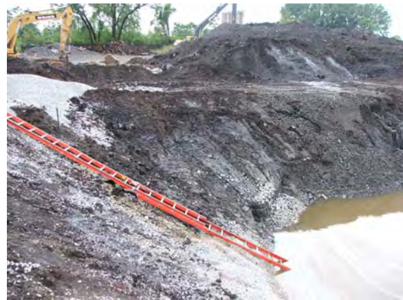
Flooded central sump after rain event.
