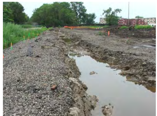
Rain water atop structural barrier wall
