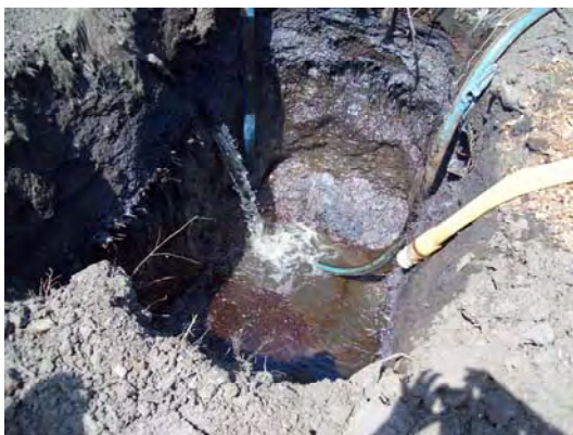
Temporary filtration system for the discharge of water.
