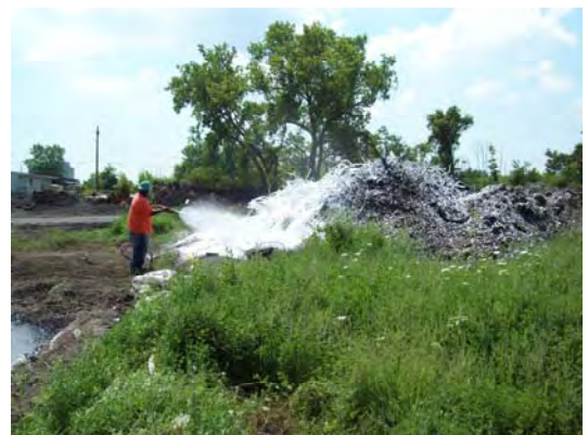
RUSTMAR odor control foam placed on top of soil and debris removed from tar well
