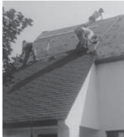
Right: Roofers strip off three layers of roofing to make way for the original style 3-tab shingles used in 1917. An historic easement will result in a permanent 15% reduction of the property tax.
