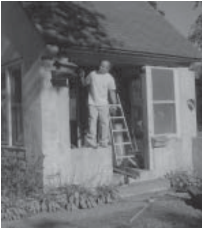
Left: Rafael Bejar opens up the front porch of a recently acquired property and in doing so increases the security of the building and guarantees a property tax reduction for the home.
