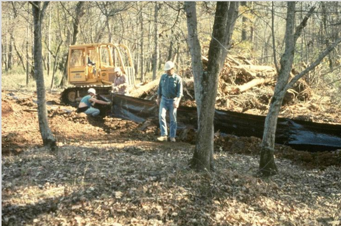
Workers installing a silt fence. Source: In Stream Corridor Restoration: Principles, Processes, and Practices (10/98). By the Federal Integrity Stream Restoration Working Group (FISRWG)
