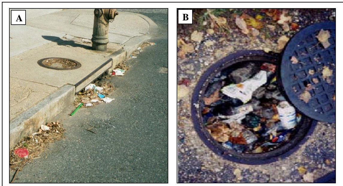
Figure 37: Envisioning Restoration on Streets and Storm Drain Inlets Pollutants and trash can accumulate on street surfaces and curbs (Panel A) or within storm drain catch basins and sumps (Panel B). Street sweeping and catch basin cleanouts may be the last chance to remove these pollutants in highly urban subwatersheds with few other restoration options.
