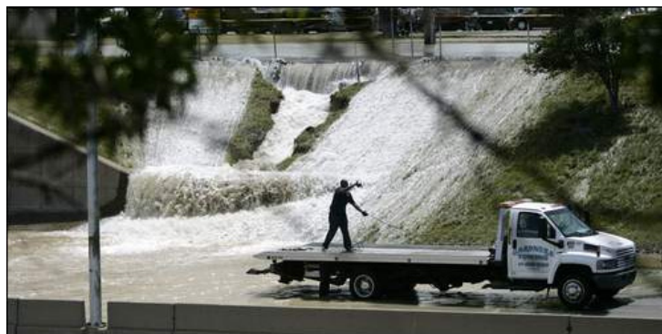
Figure 5. Broken water main along I-96 freeway Photo by: John T. Greilick
