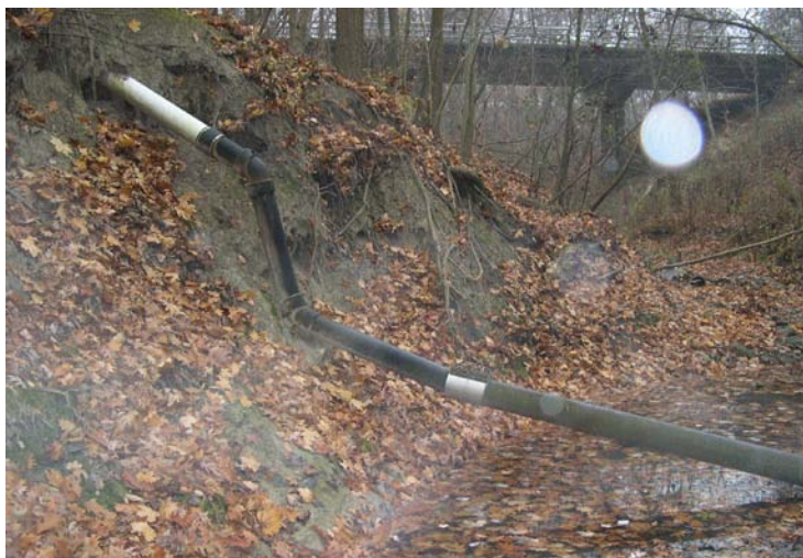
Figure 9. Recent repairs to an undercut, leaking sewer line at a stream crossing in Lake County, Illinois Photo by: Michael Adams, 2007
