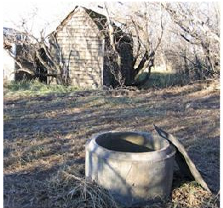
Figure 3. Improperly covered well Source: Jones, 2006
