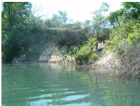
Figure 4: Bank erosion at Ambridge Park.
