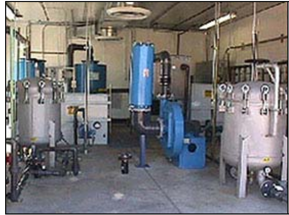
Groundwater treatment center. Source: http://www.tucsonaz.gov/ets/Groundwater/Los_Reales/los_reales.html
