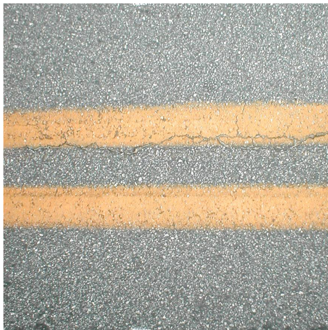
FIGURE 1-1 Photograph of double yellow line in the center of a road, Emory University campus, Atlanta Georgia. Window size (extent) of photograph is 1 m \times 1 m. Source: Photograph by L. Gunderson.
