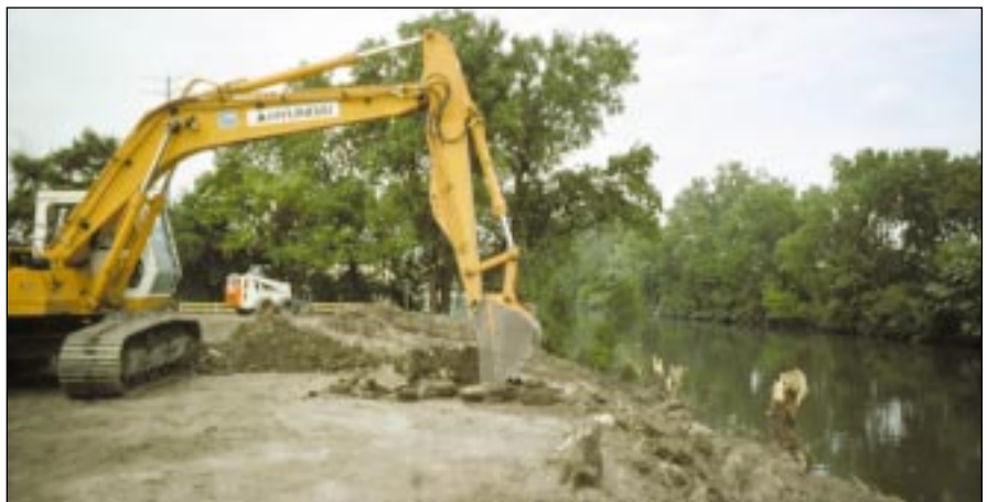
A local contractor, working with CYC Fellowship House, completed an extensive re-grading of the riverbank, successfully stabilizing the highly erodable soils. Courtesy of dr/Balti Contracting Co., Inc.
