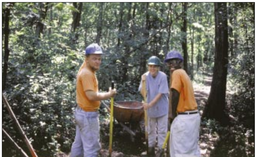
Members of the Lake County Youth Conservation Corps installing a boardwalk along portions of the trail. Courtesy of Lake County Forest Preserves.
