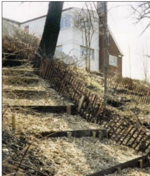
Terraces built in the steep riverbank reduced soil erosion and enabled the establishment of vegetation. Courtesy of Pete Leki.
