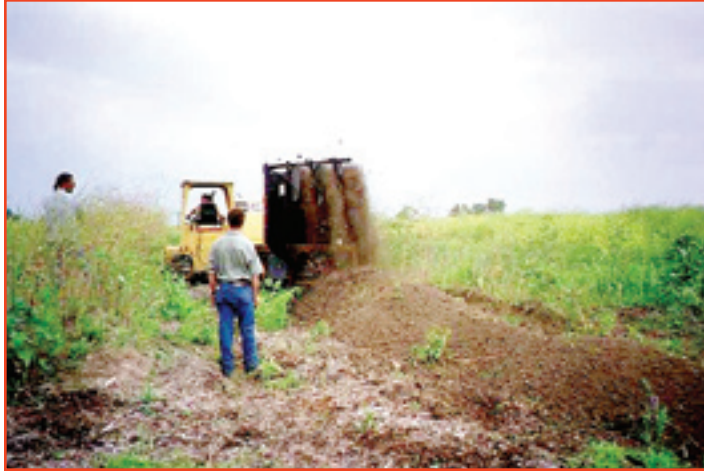
Mixing dredged material with biosolids and woodchips at Milwaukee CDF. Credit: U.S. Army Corps of Engineers
