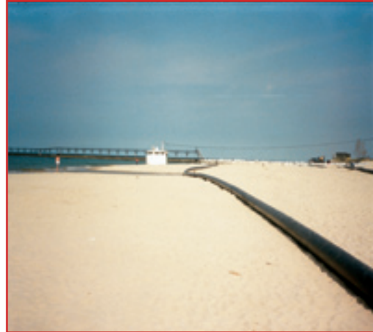
Beach nourishment at Grand Haven, Michigan. Credit: U.S. Army Corps of Engineers
