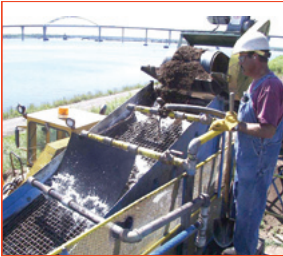
Sediment separation plant in operation at Erie Pier CDF Credit: U.S. Army Corps of Engineers
