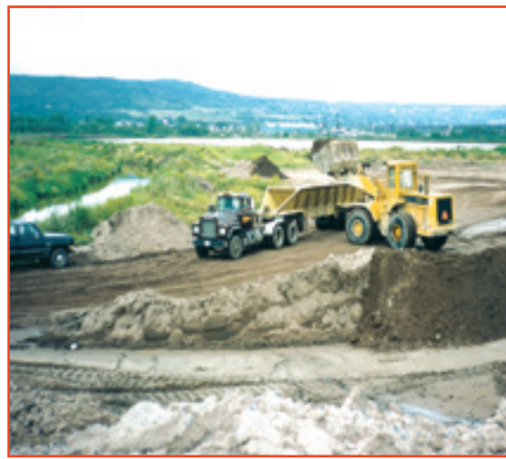
Construction fill being loaded at Erie Pier CDF Credit: U.S. Army Corps of Engineers
