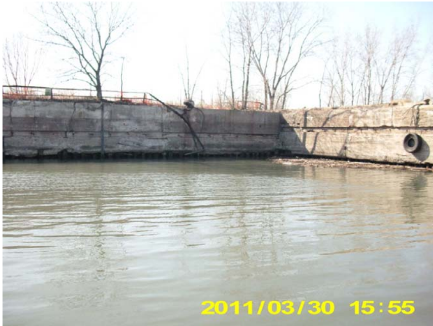
Photo 5. South Slip looking northeast from a barge within the slip towards the timber-supported concrete dock. March 30, 2011.
