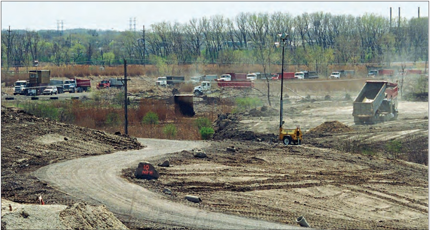
Parade of trucks carries excavated soil from the Illinois Department of Transportation's Dan Ryan Expressway Reconstruction Project for use in capping the Lake Calumet Cluster Sites.
