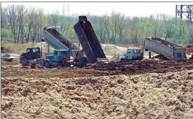
Soil from the Dan Ryan Project is stockpiled at the Paxton I site for use in the Cluster Sites capping remedy.
