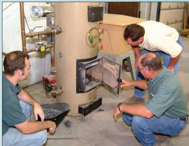
P2 intern Eric White (left) discusses his project to incorporate an air-conditioning cycle with the corn burning boiler units made by Big M Manufacturing in Taylorville, with owner Melvin Repscher (center) and Brian Rodely of the IEPA Marion Regional Office
