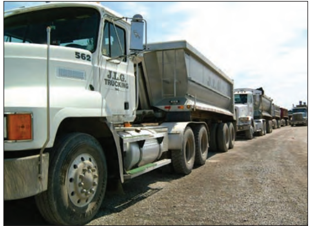
Hundreds of trucks line up to drop their loads of soil from the IDOT Dan Ryan Expressway Reconstruction Project for use as cover in the remediation of the former Paxton I waste disposal area.
