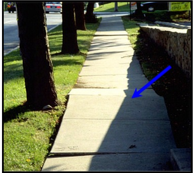
Figure 9. A common infrastructure conflict results in tree roots lifting or cracking pavement due to inadequate setbacks between trees and pavement (Photo by Ed Gilman)
