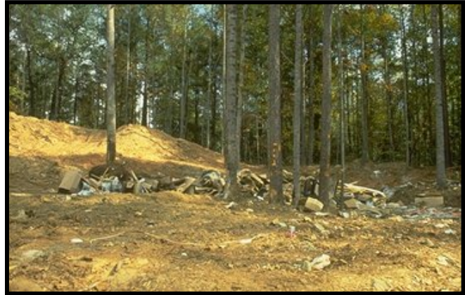
Figure 6. Improper disposal of construction materials and inadequate protection have impacted trees at this construction site
