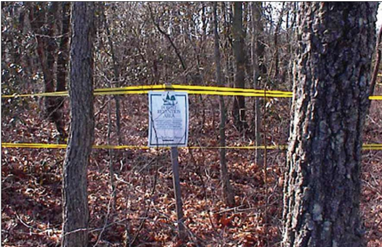
Figure 15. Sign posted at construction site informs workers of forest protection area.
