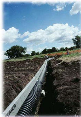
Coffee Creek, Chesterton: the photo on the top shows level spreader water filtration process, which the stormwater is taken into the underground pipe system. When a pipe is full, the water will seep through the grate and flow over the ground as shown on the above picture.
