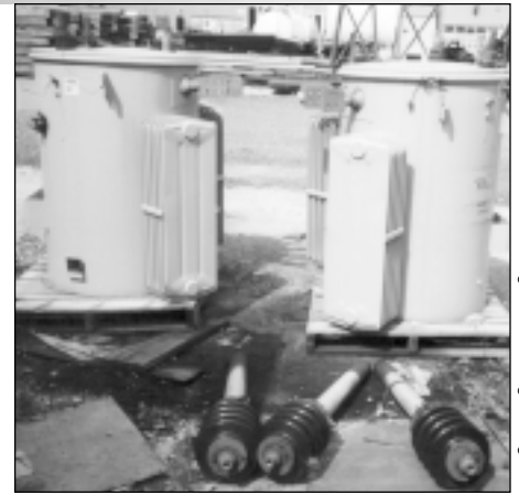
Transformer Storage Yard – Ying-Kuang Hsu
