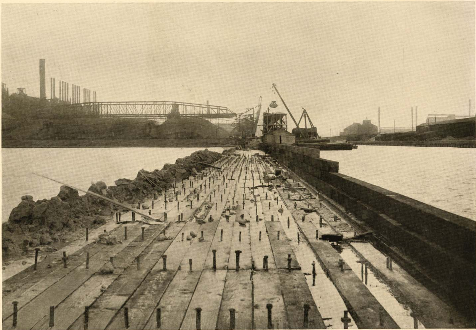
SOUTH CHICAGO, ILLINOIS: Crib work ready for concrete superstructure, built for the Illinois Steel Company's plant on Calumet River.
