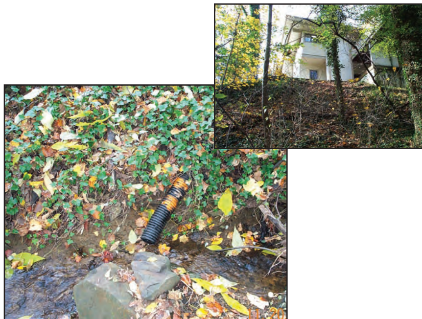
Figure 25: The origin of this corrugated plastic pipe was determined to be a roof leader from the house up the hill.
