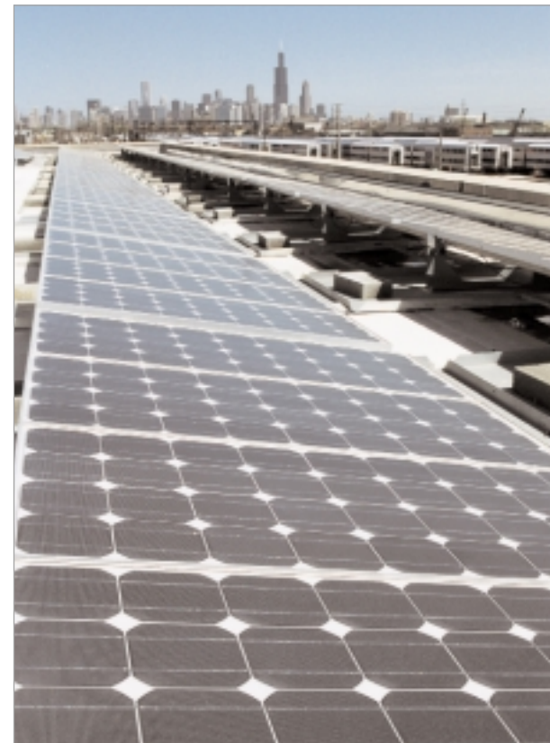
Solar panels along the CCGT building's roof
