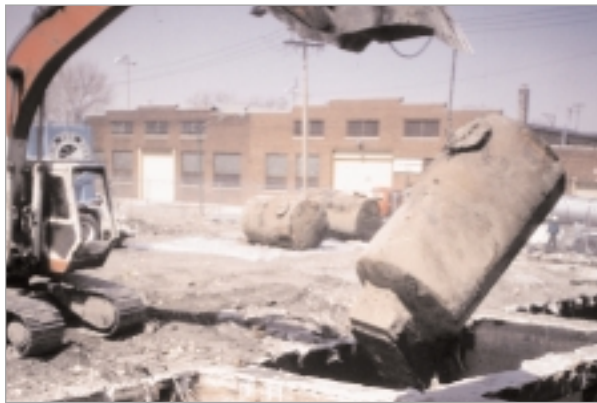
Underground storage tank being removed from site Above right: The new ATA training center will inject new life into the area
