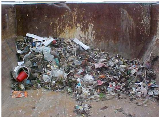
Floatable material collected on the intakes screens of the Midwest Generation's Crawford Station.
