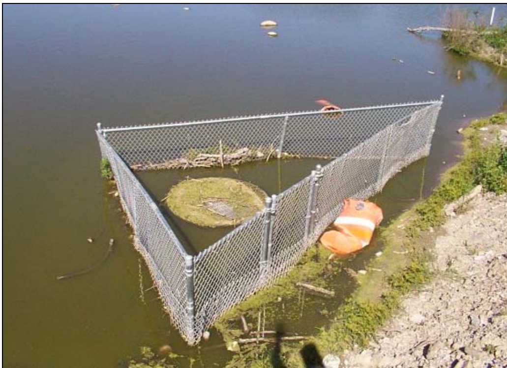
Figure 11: Structure #3 - Obstructed Gate.
