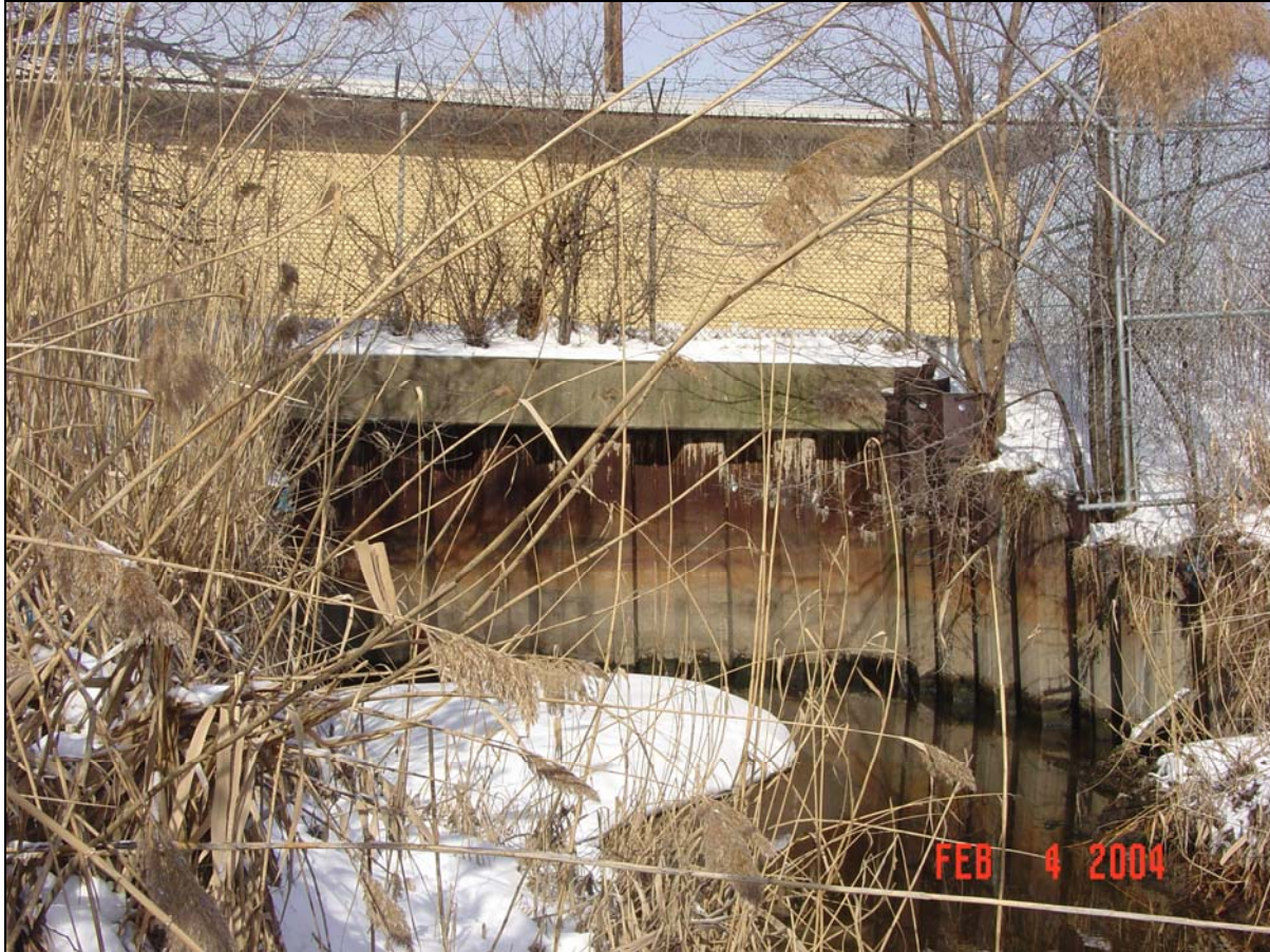
Figure 2: Pump Station Discharge to Outlet Channel.
