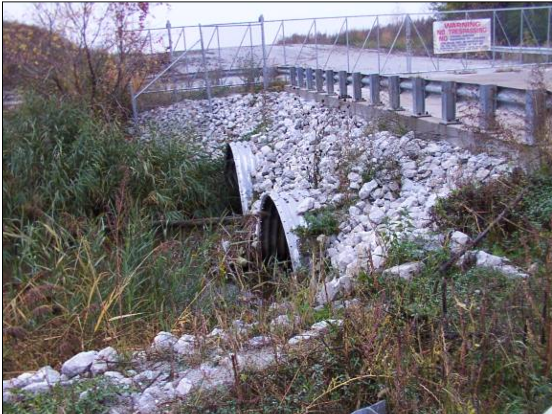
Figure 24: Structure #9 – Pullman Creek Double Arch CMP Culverts Under Illinois International Port District Driveway at 116 th Street.
