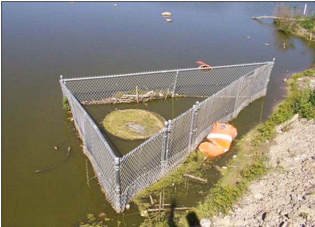
Figure 15 – Structure #3 Obstructed Grate.
