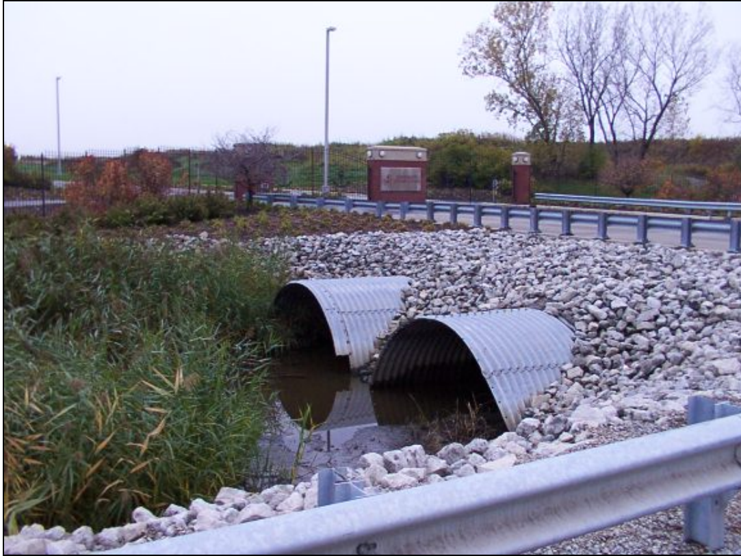
Figure 25: Structure #10 – Pullman Creek Double Arch CMP Culverts Under Harborside International Golf Course Driveway at 111 th Street.
