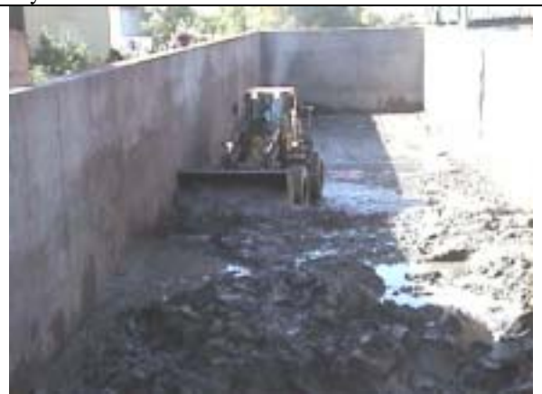
Fig. 8. Later in the day an endloader inside the barge pushed material into a pile to assist the excavator.
