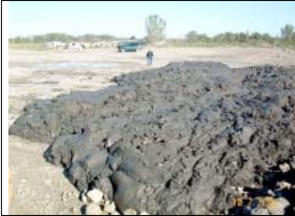
Fig. 21. Trucks were able unload sediment in contiguous piles demonstrating the ability to form a continuous layer about two feet thick.
