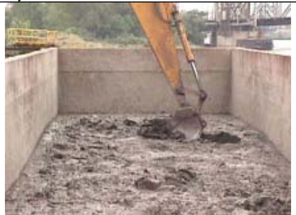
Fig. 6. A three cubic yard excavator removing sediment from the barge. The top layer has begun to dry and form a thin crust.
