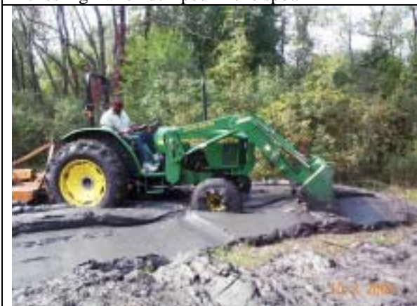
Fig. 13. The material was stiff enough to allow an endloader to spread it without using a form.
