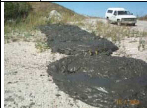
Fig. 23. Sediment stayed in place along the side of the roadway leading up the landfill flowed only a few inches downhill. The slope is 8%.
