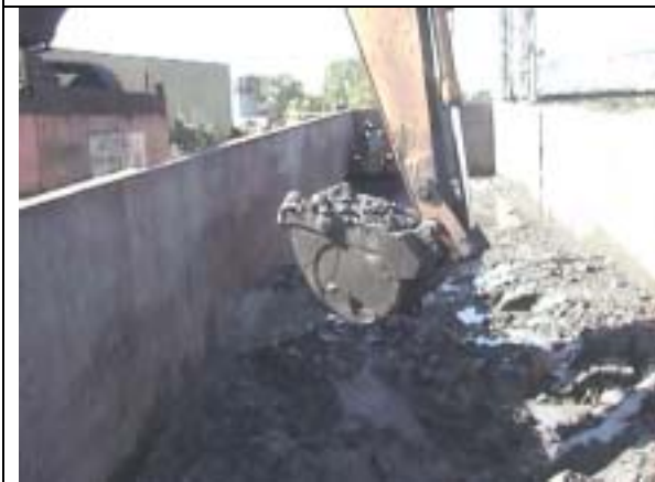
Fig. 7. The dredged material handled well in the bucket and maintained its consistency.
