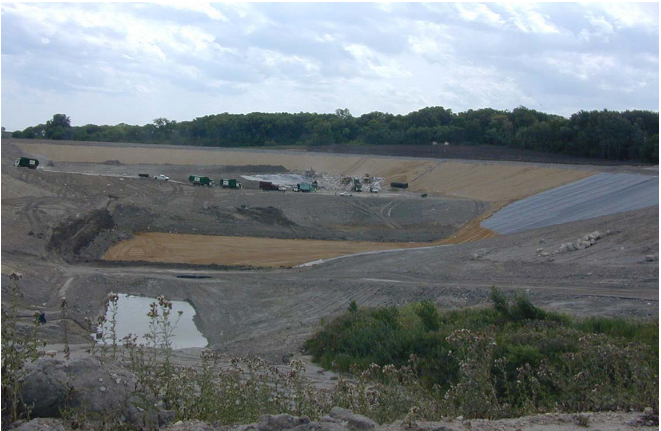
Cell 5B (foreground) at Countryside Landfill, Grayslake, underwent excavation which allowed the landfill operator to stock pile soil to be used as daily cover in the active fill operation (Cell 5A) (background).
