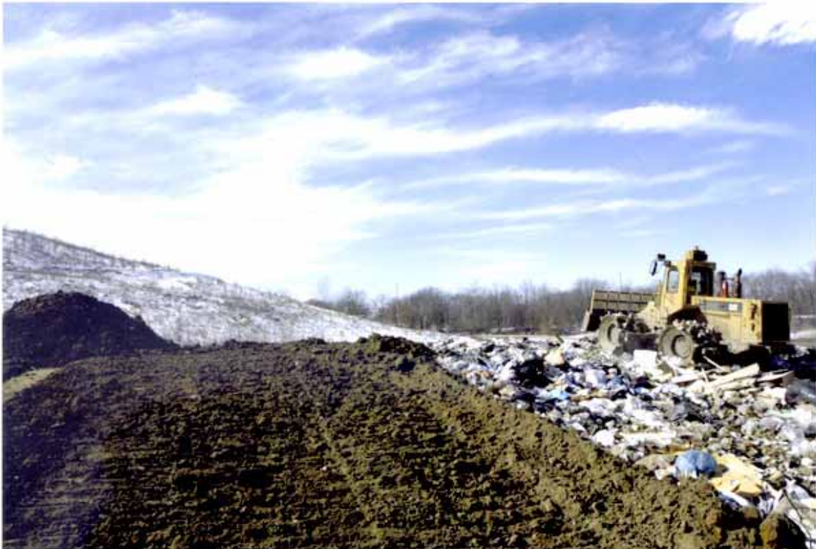
Sangamon Valley Landfill, Springfield re-opened in July 2003 after remedial efforts were accomplished by its new owner/operator.
