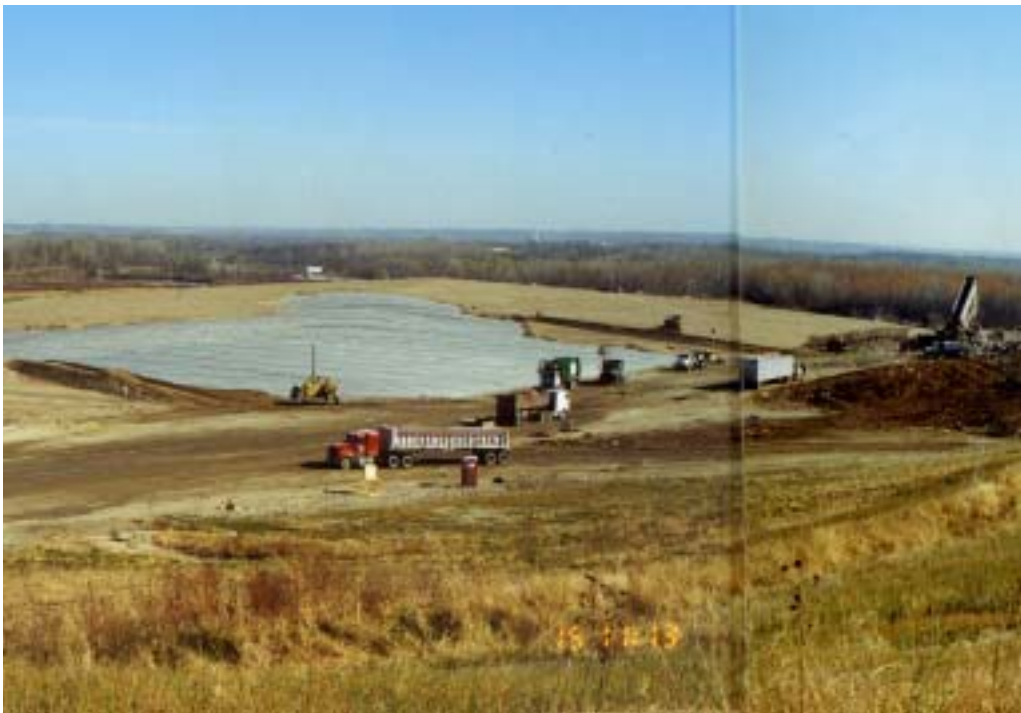
Milam RDF, East St. Louis ranks #5 in the State for wastes disposed (44 percent of the receipts disposed in Region 6)
